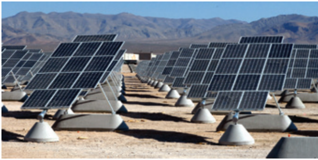
Figure 1. A photovoltaic array at Nellis Air Force Base, Nevada. The 15-megawatt array installed in 2007 currently provides 25 percent of the base's energy needs. (Photo courtesy of Nellis Air Force Base.)
